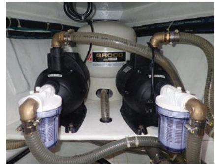
Two fresh water pumps adds redundancy.
